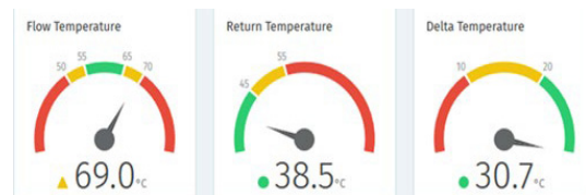
70°C flow and 40°C return temperatures at the energy centre
